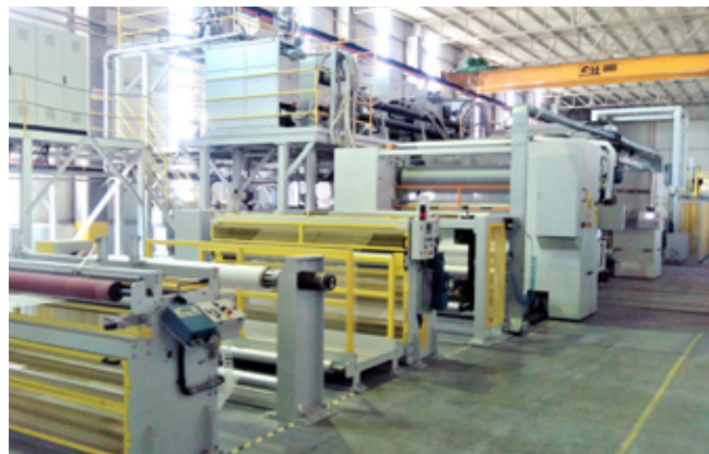
Processing raw materials into premium quality membranes by way of flat-die coextrusion.
